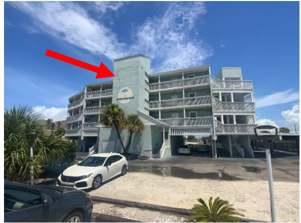
Photo 23 View of rippling effect at direct applied stucco at elevator tower.
