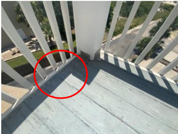
Photo 20 View of isolated corroded fasteners at treads.
