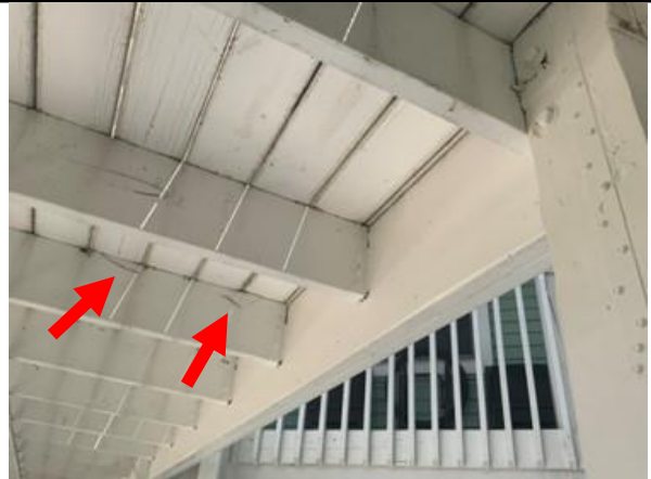
Photo 22 View of isolated cracked joist at walkway.
