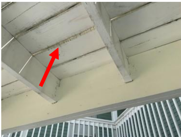
Photo 21 View of isolated split deck board.
