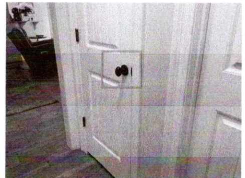
Closet door in hallway does not latch
