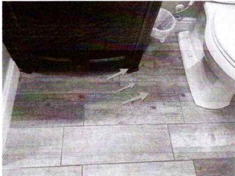
Cracked tile here
