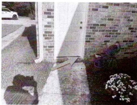
Some wood rot here
