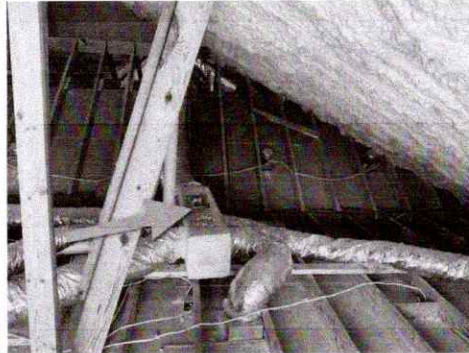
Open vent here
